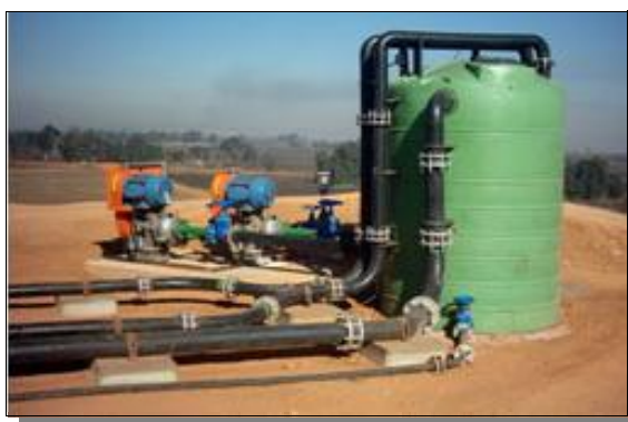
Balancing tank and return water pumping system on the wall of the facility
