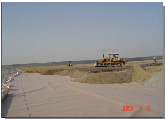
Prior to placing the protective soil cover, a Secutex geotextile was placed over the Carbofol
