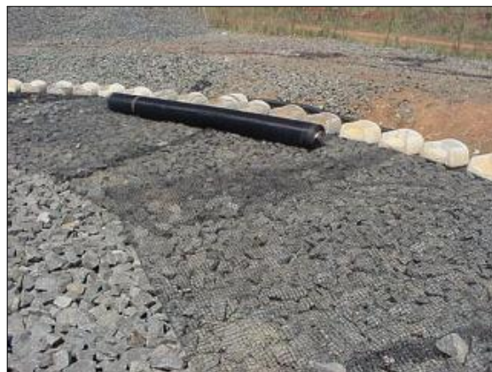
The biofilter at the Delmas Waste Water treatment works in Mpumalanga was the first to be built using Kaytech's Rock GX
